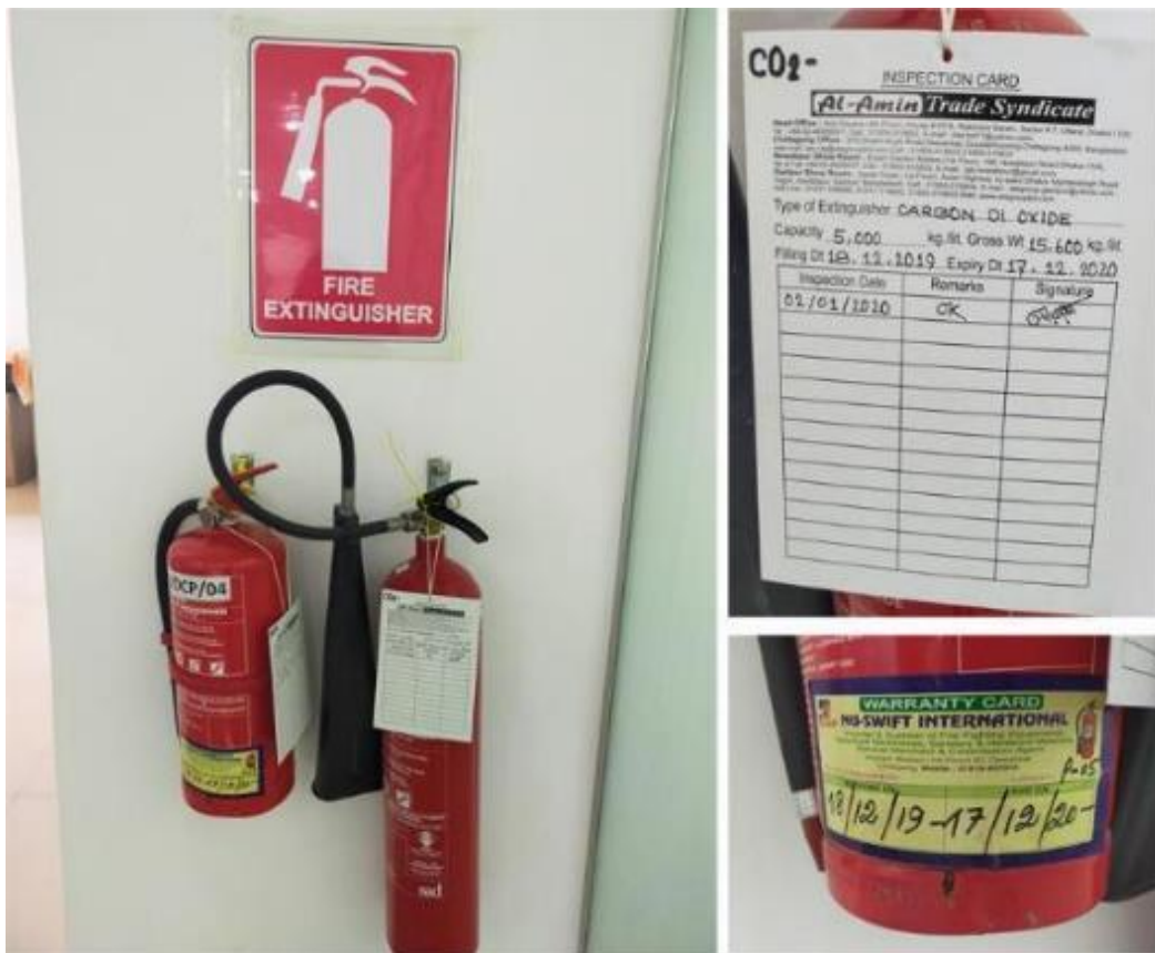
Photo 26: Fire Extinguisher and Updated Inspection Card
