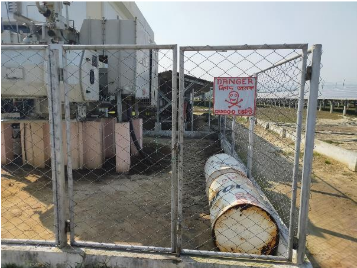
Photo 14: Caution Signs In Restricted Places inside the Plant
