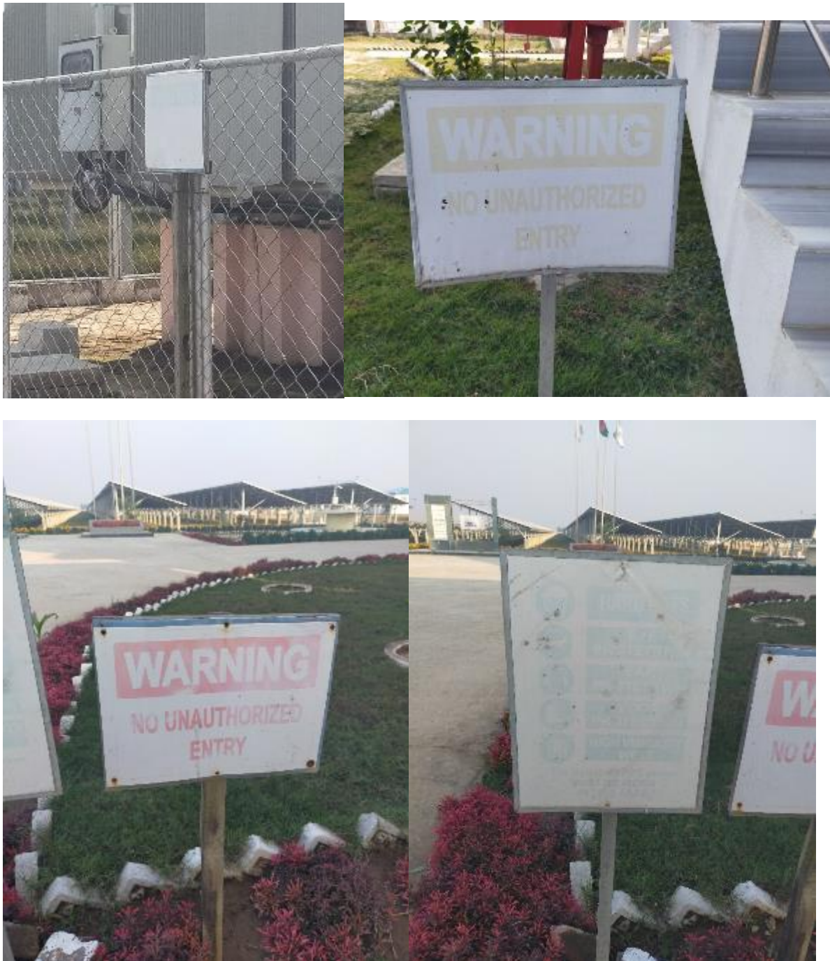
Photo 15: Faded Sign Board that needs to be replaced
